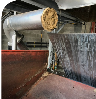
Discharging spent grain from AWP
