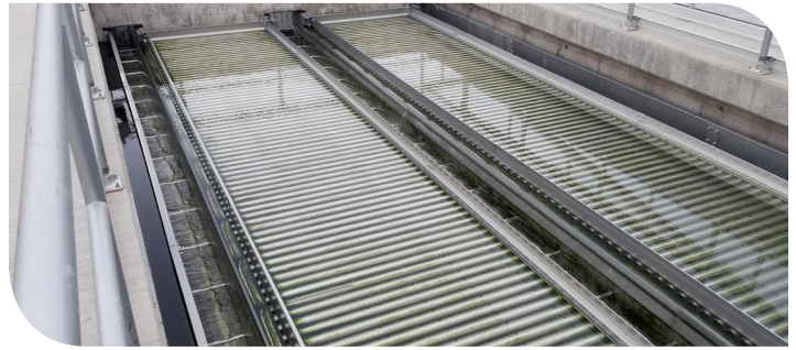
MRI Inclined Plate Settlers installed at Tri-Lakes WWTF
