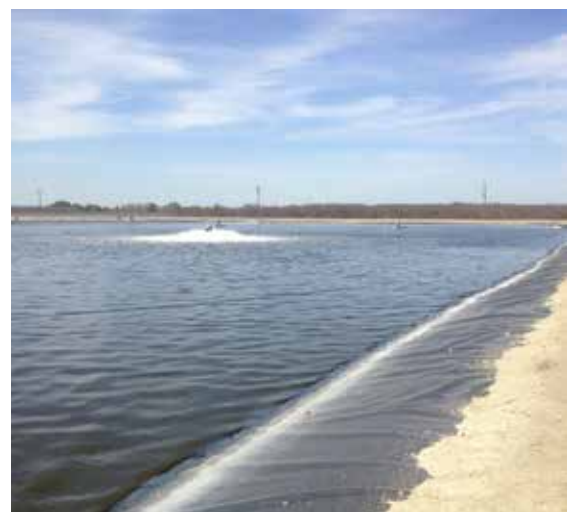
Figure 4: Surface Aerator (in operation)
