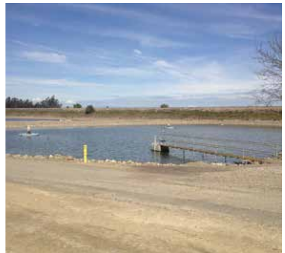
Figure 3: Surface Aerator (idle)
