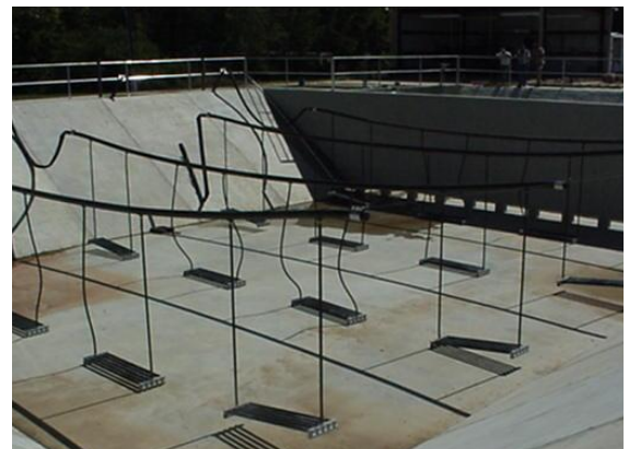
Figure 6: Aeration Chain + Diffuser
